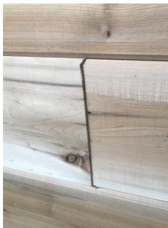
Vertical joint not flush
