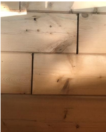
Vertical joint not kept tight
